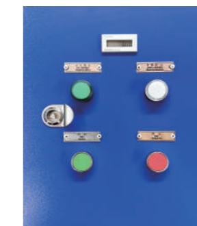
Mechanical control panel
